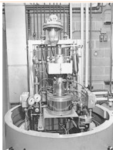
Storage Tanks and Process Tanks (4 Products)
